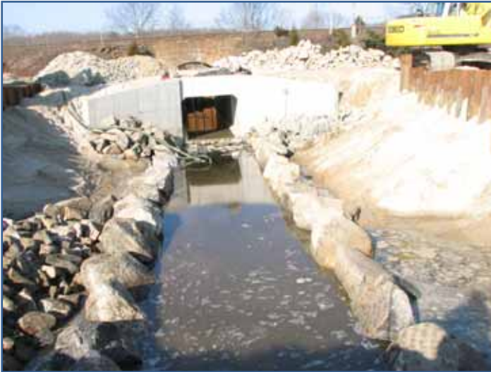
Cofferdams were used to keep the water out of the construction site as workers dug the trench and lined it with rocks. Natural sand dunes were recreated on top of the culvert. Bride Brook is now flowing through the completed channel.
