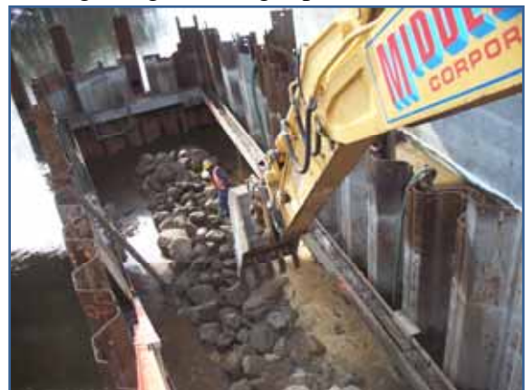
Installation of a rock reef atop the location of the removed pier in the Farmington River.
