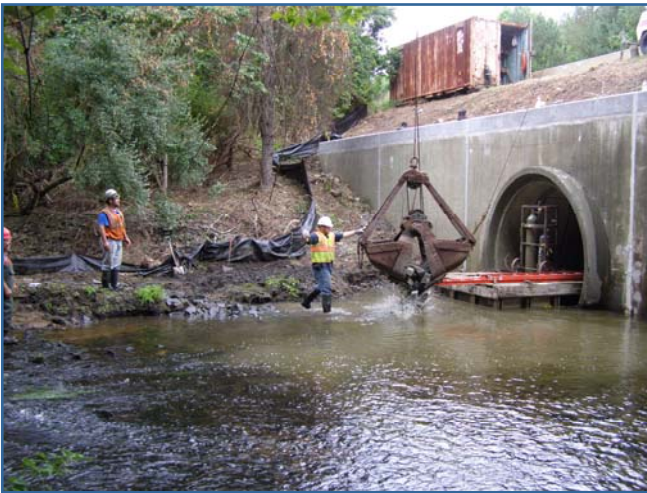
Installation of a rock vane in the Five Mile River, New Canaan.
